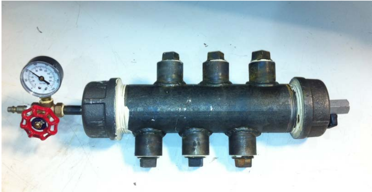
Figure 1: Corrosion Coupon Testing Manifold.
